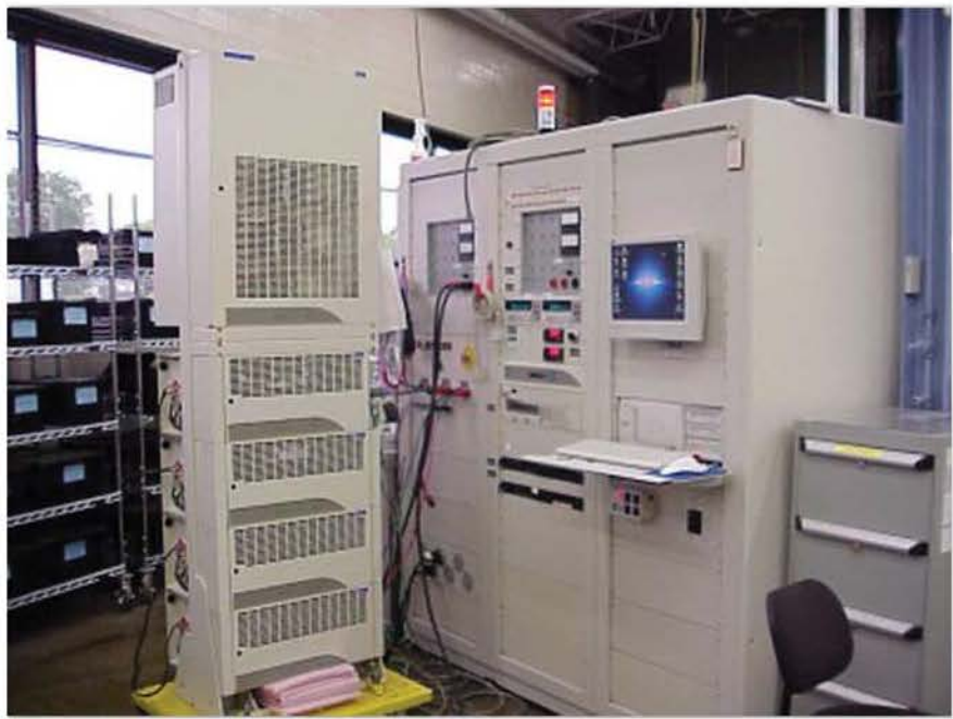
Manual Tester #1 with a Power Cabinet Connected
