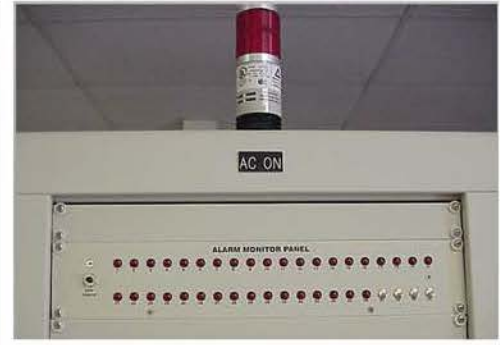
Flashing Lamp and UUT Alarm Panel
